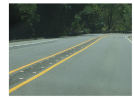
MEDIAN RUMBLE STRIP EXAMPLE
